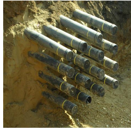
150 kV power line, Switzerland
