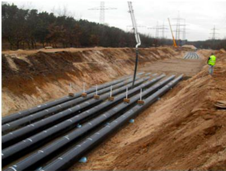
420 kV GIL-Line by Siemens
