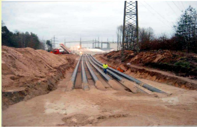
420 kV GIL-Line by Siemens (gas-isolated lines)
