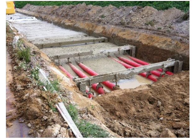
Amprion 380 kV line in Raesfeld
