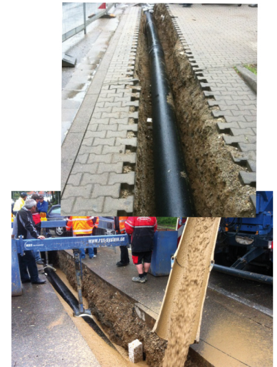
District heating pipe
