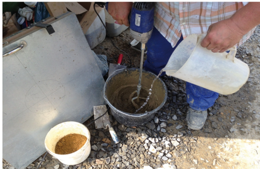
Preparation of a "bucket mixture" of RSS Flüssigboden® for the determination of the cubature
