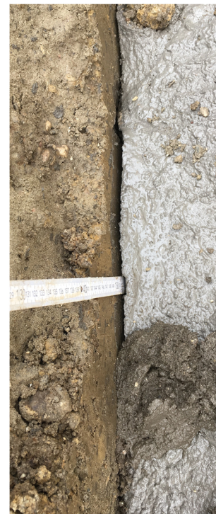
Torn off block
